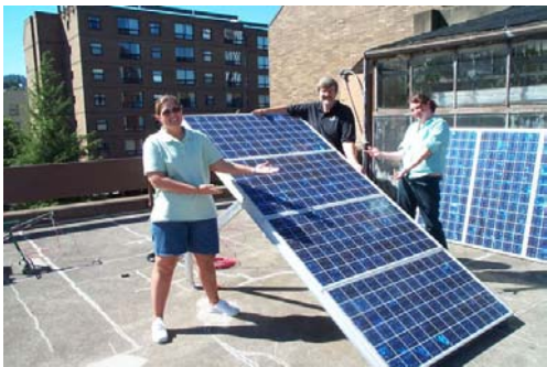
Students in Carl Wamser's 2001 summer course on solar energy assisted with the assembly and installation of a 1 KW photovoltaic system
