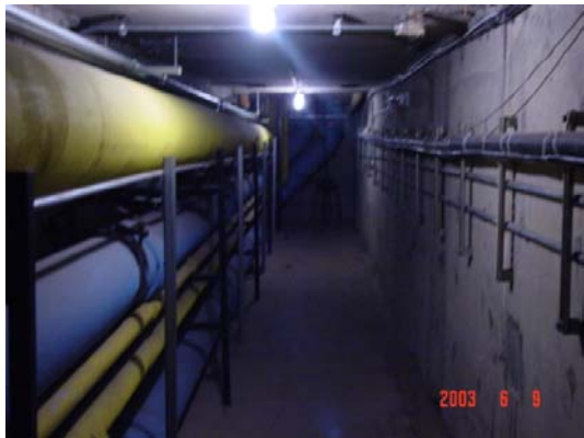
The "Tunnel" – PSU's underground energy distribution system
