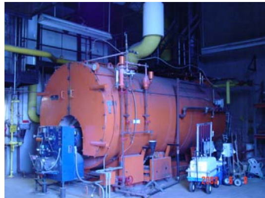
The West Heating Plant's Kawancee Boiler, installed 1972
